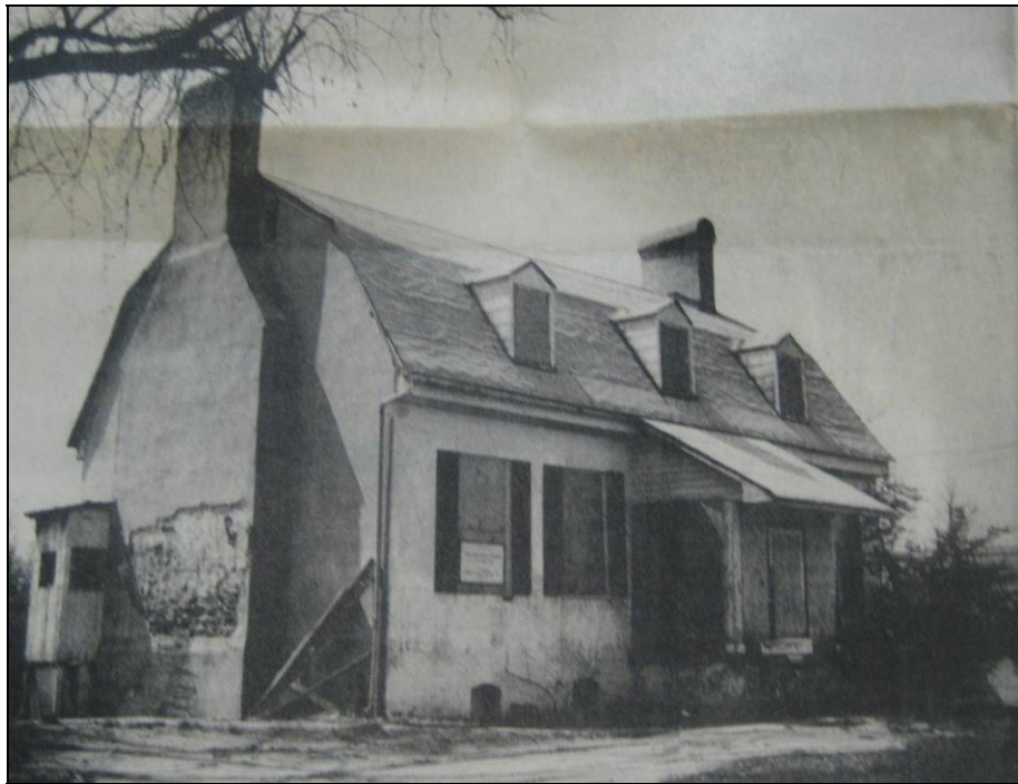
Figure 32: The Magruder House prior to the 1982 Restoration Source: Prince George's Journal/PGCHS Library
