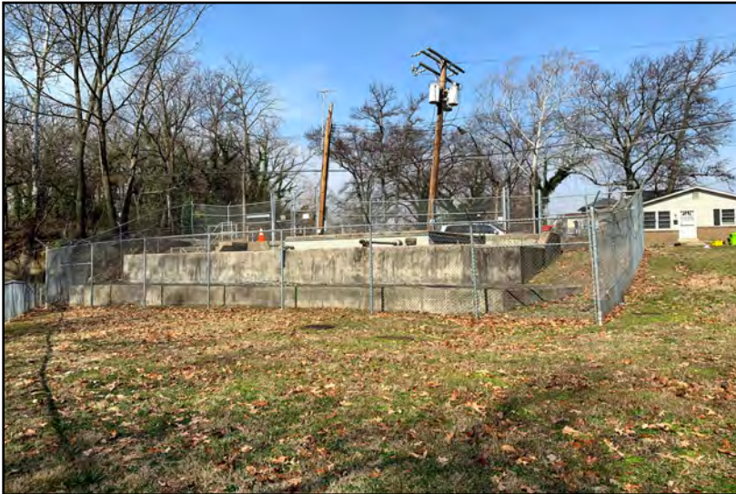
WSSC Pumping Station
